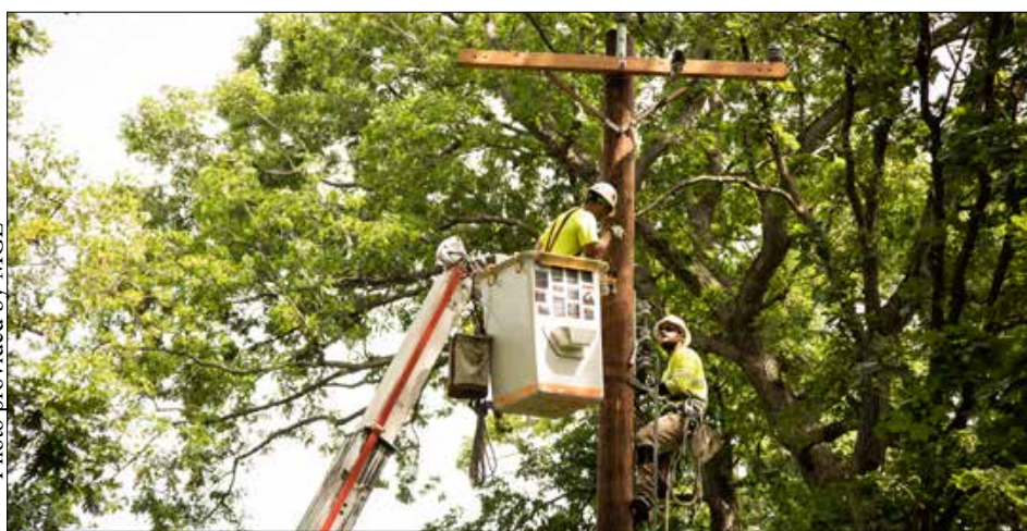
MGE is upgrading the Northside electric system in 2024
