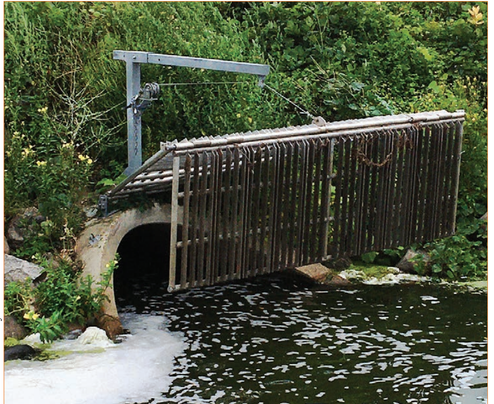
The carp gate at Warner Pond can be raised and lowered.
