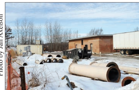
The wastewater pumping station at Cherokee Marsh’s South Unit is getting new pumps, pipes and other upgrades.
